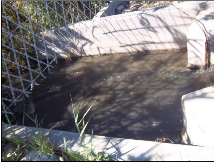
FIGURE 8: DIRTY SEWAGE EFFLUENT RUNNING INTO THE BLES SPRUIT
