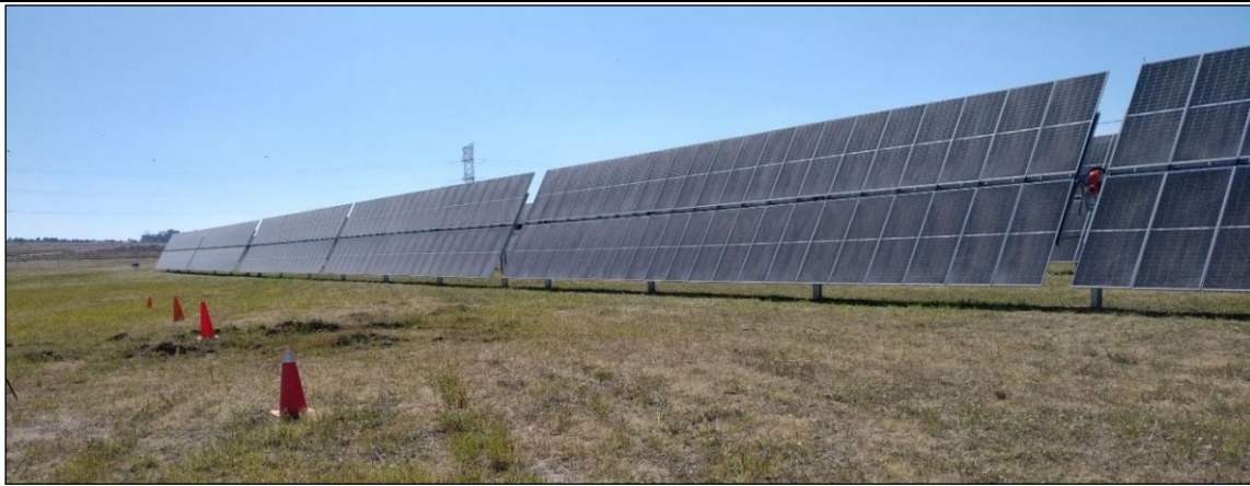
Figure 4.4: Frontal view of PV arrays mounted on fixed mounting systems.
