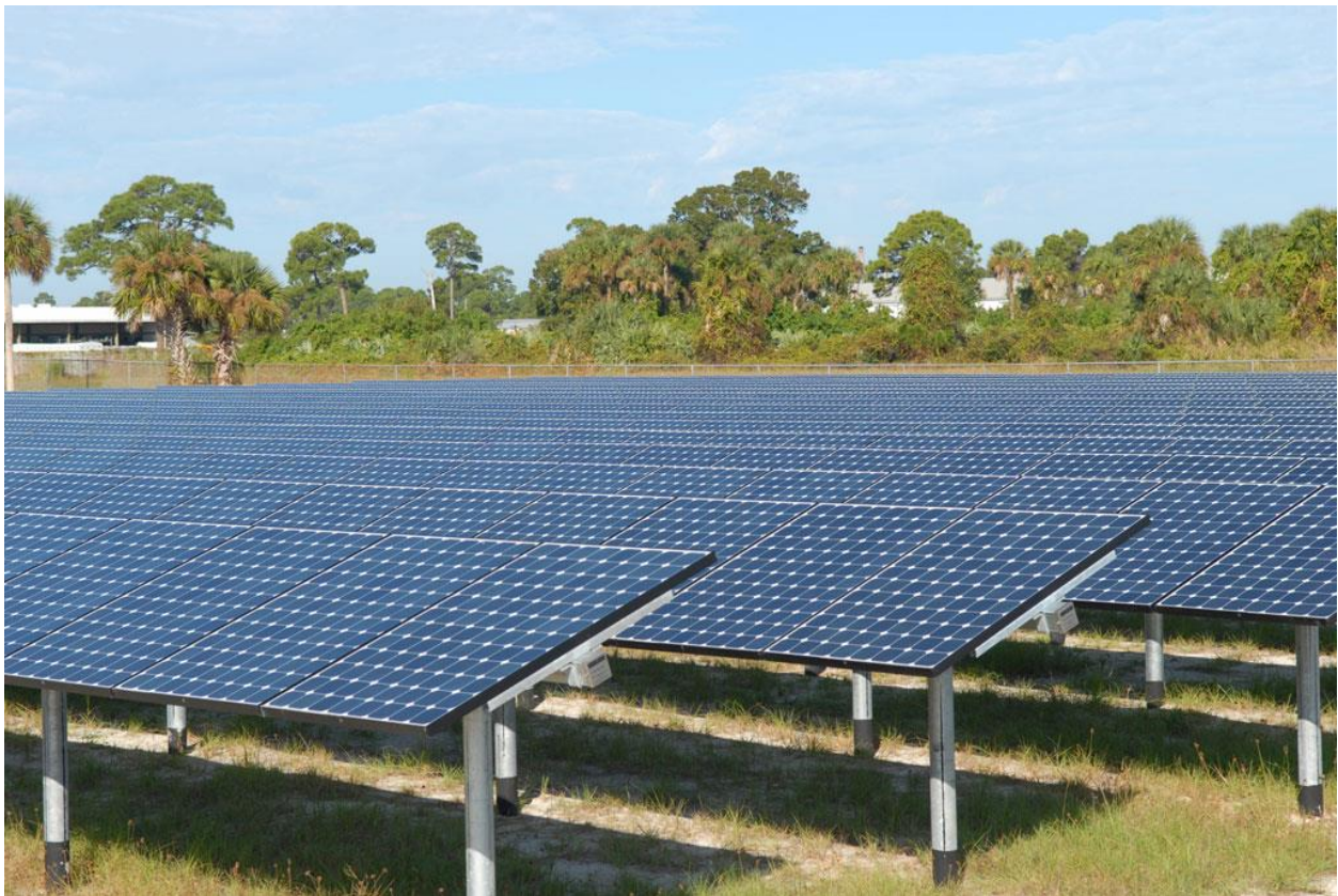
Figure 2-4: Photovoltaic (fixed-tilt/ static) panel array
