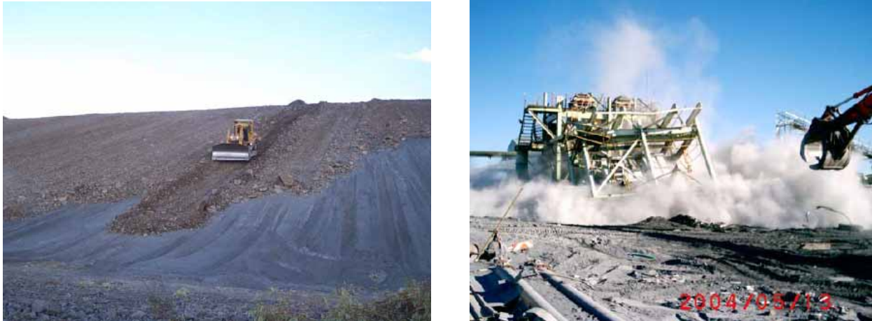
Figure 4: Activities undertaken at closure (rock cladding of tailings dam and plant demolition)
