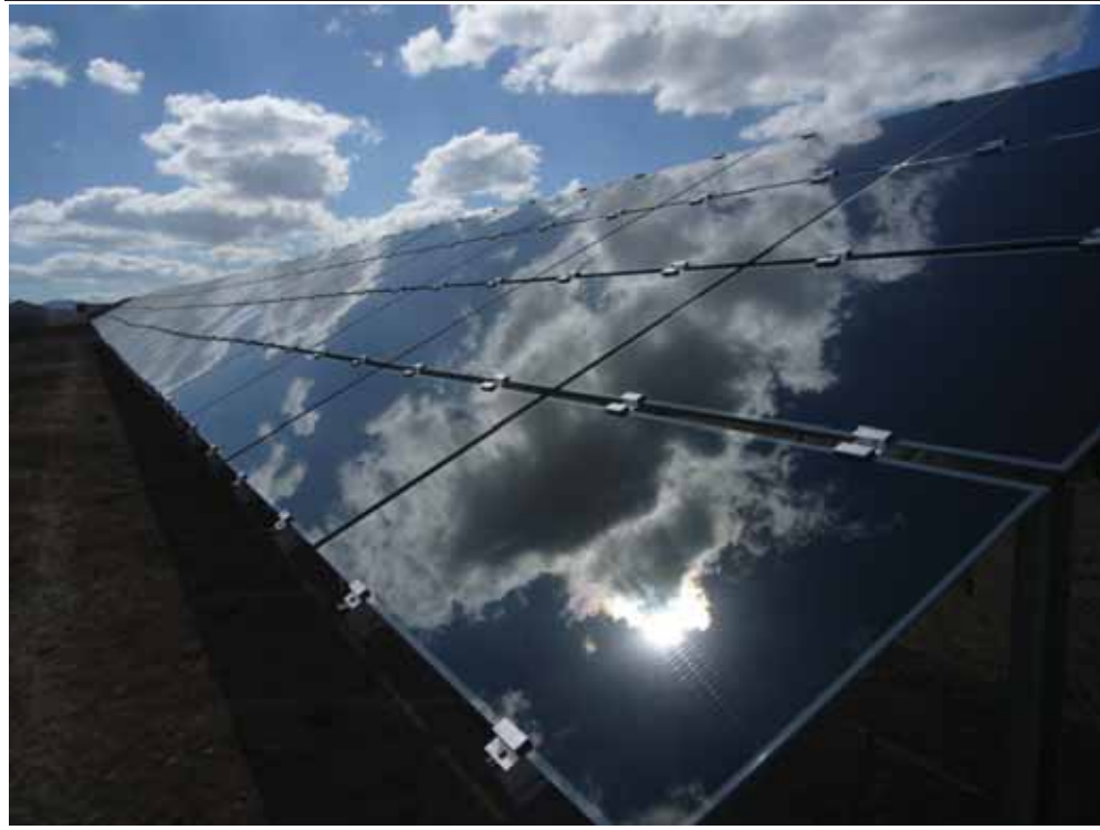
Figure 4.4 Typical PV Array
