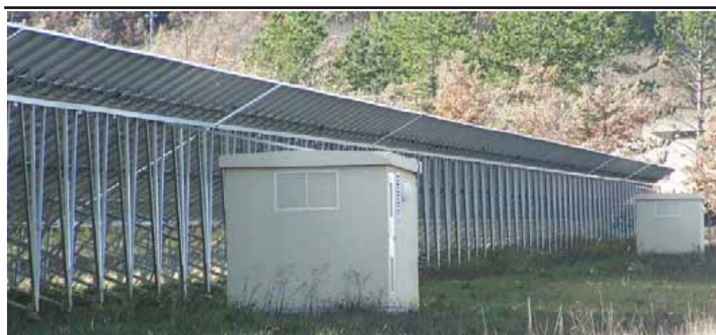
Figure 4.7 Typical Inverter/Transformer Enclosures
