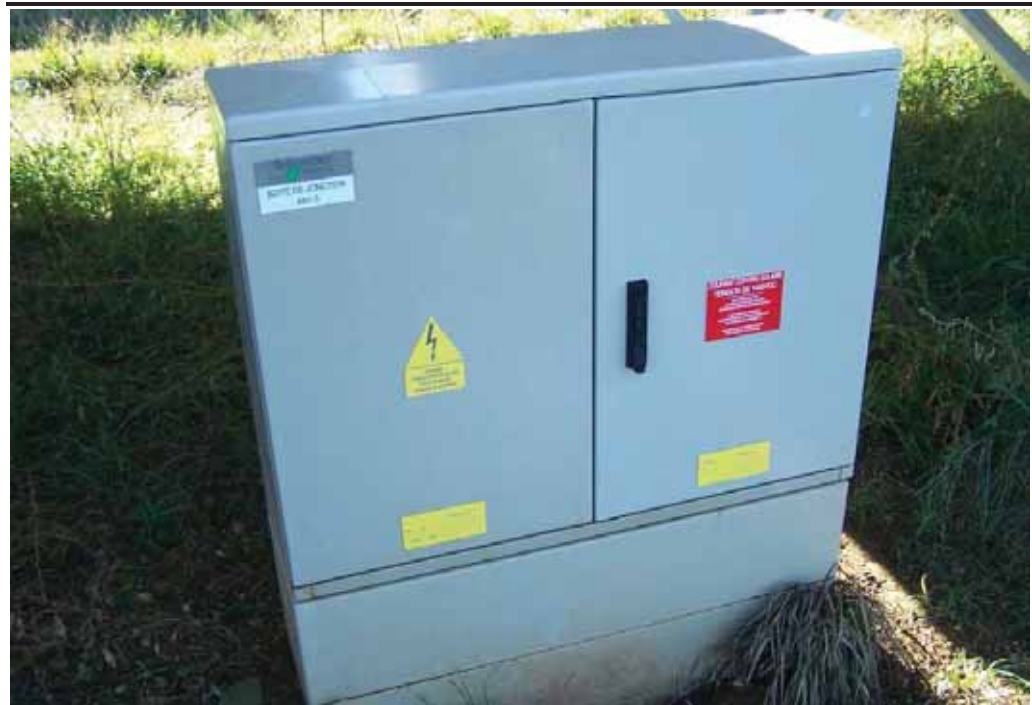
Figure 4.5 Typical Array Enclosure
