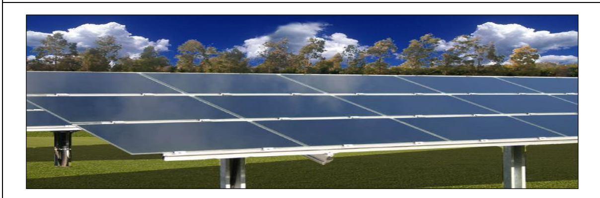
Figure 5-3. Frontal views of PV arrays mounted on fixed mounting systems.
