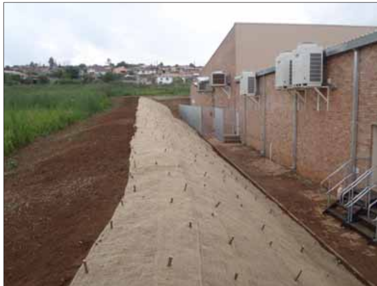
Figure 7-9 An example of the use of 'Bio-jute' in a newly worked area
