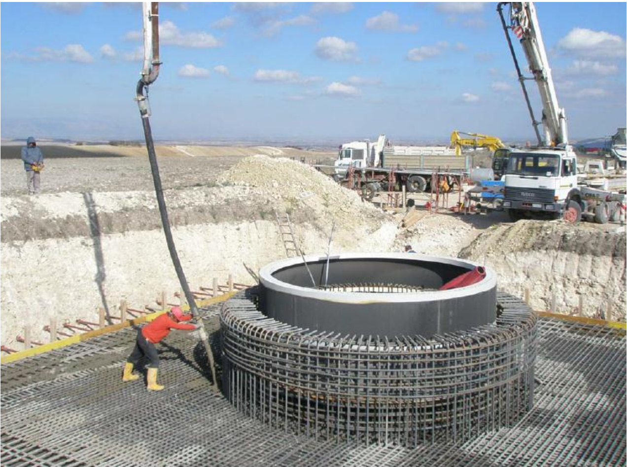
Plate 2-2: Concrete pouring of a turbine foundation – note the tower base collar in the foreground.
