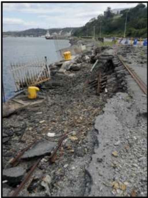
Figure 4: The ferry landing is a sheet pile wall constructed in the 1900s.
