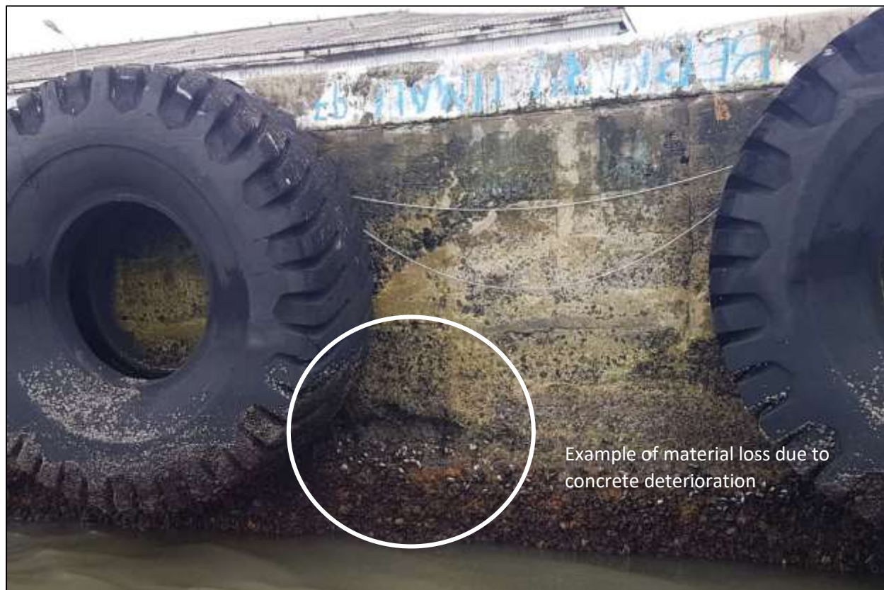
Figure 6: Example of material loss due to concrete deterioration
