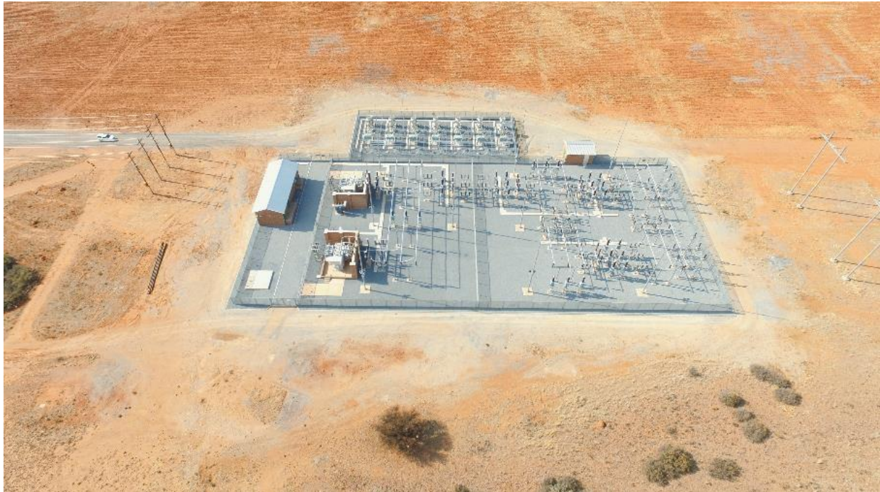
Plate 2 Lesedi Substation and Capacitor banks (during construction)
