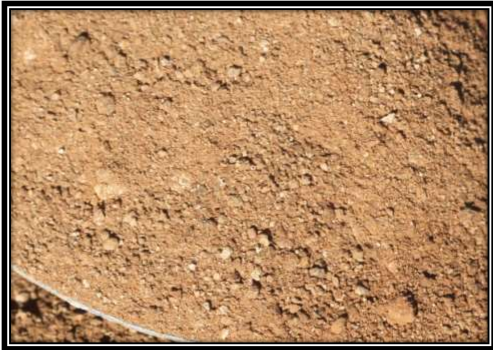
Photograph 18 Soil at bare area where erosion and poor recovery of vegetation are visible, at the site. Photo: R.F. Terblanche
