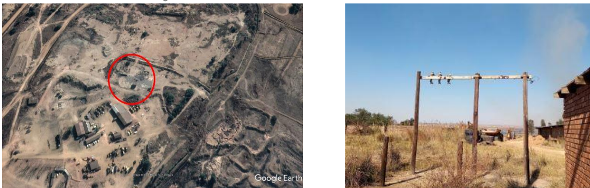
Figure 5: Decommissioned Eskom Supply Point on the proposed site
