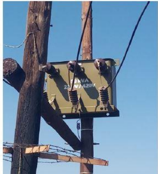
Figure 3: Eskom Pole BRI/LA3 107/13
