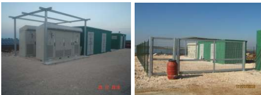
Figure 26: Typical example of on-site substation and transformer (Solek, 2013)
