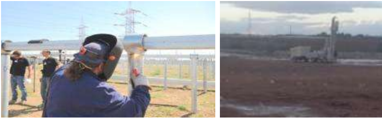
Figure 34: Showing typical erection of PV panels during the construction phase of the project (Solek, 2013).
