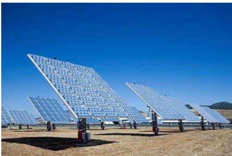
Figure 19: Example of concentrated photovoltaic (CPV) facility (Solek, 2013)
