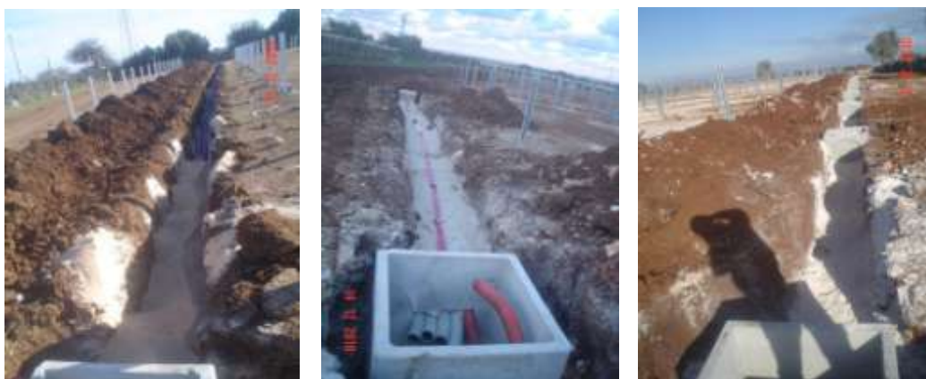
Figure 27: Examples of typical cable trenching used to connect the PV panels to the on-site substation (Solek, 2013)
