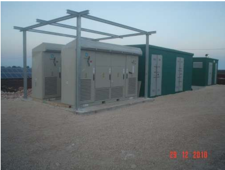
Figure 35: Showing typical example of on-site substation.
