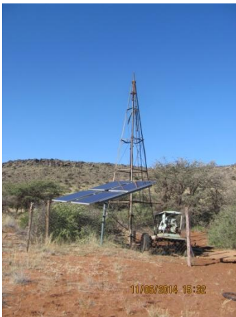
Figure 20: Solar pump and borehole.
