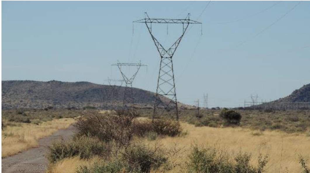
Figure 44: Existing Eskom 132kv powerline and the small substation located to the east of the project site (Stead, 2015).
