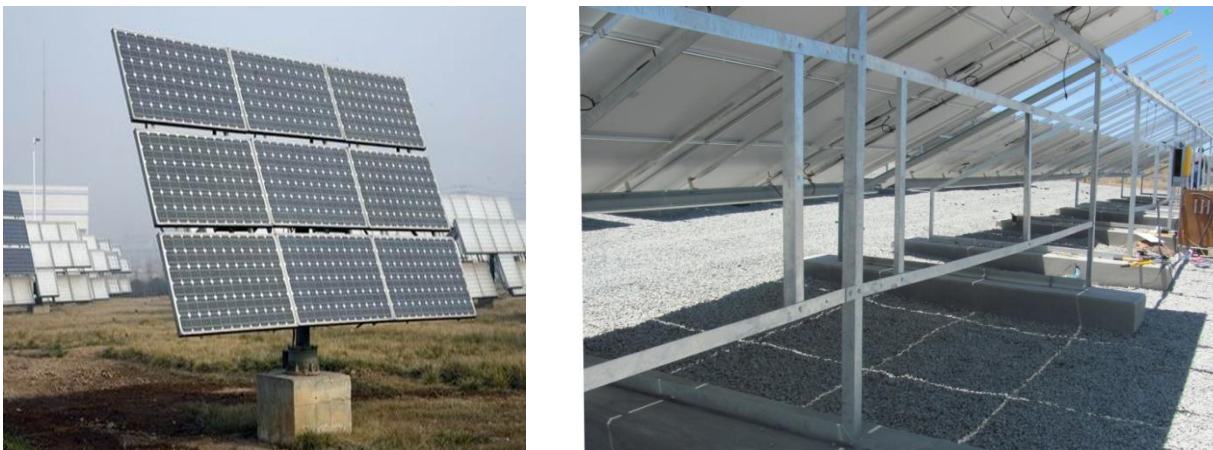
Figure 6: Examples single axis & fixed solar cast foundations.
