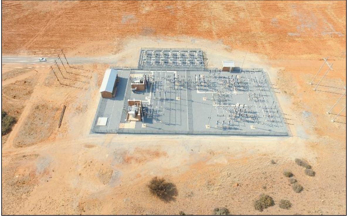
Figure 7: Substation, capacitor banks and grid connection
