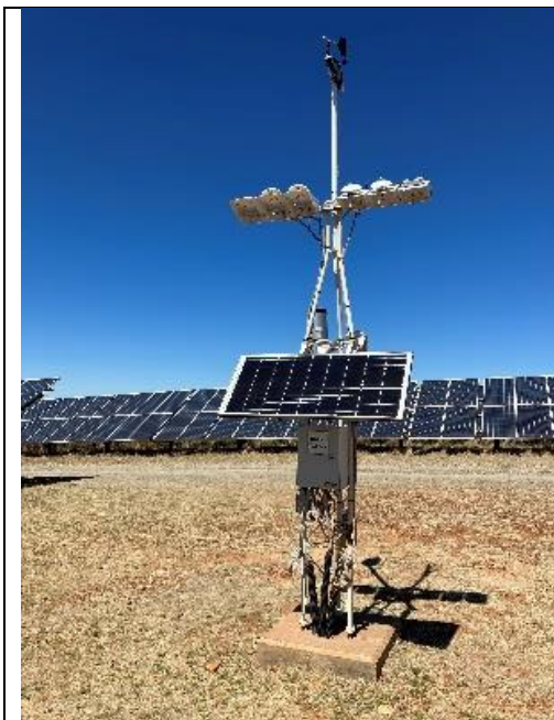
A: AWS2 installed in Lesedi south solar field.
