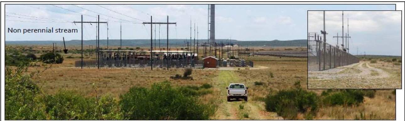
Figure 36: View of the substation, looking northwards, in a grass dominated landscape (Vegetation Review, 2023)
