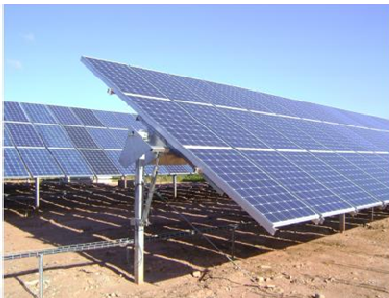
Figure 3: PV panels installed
