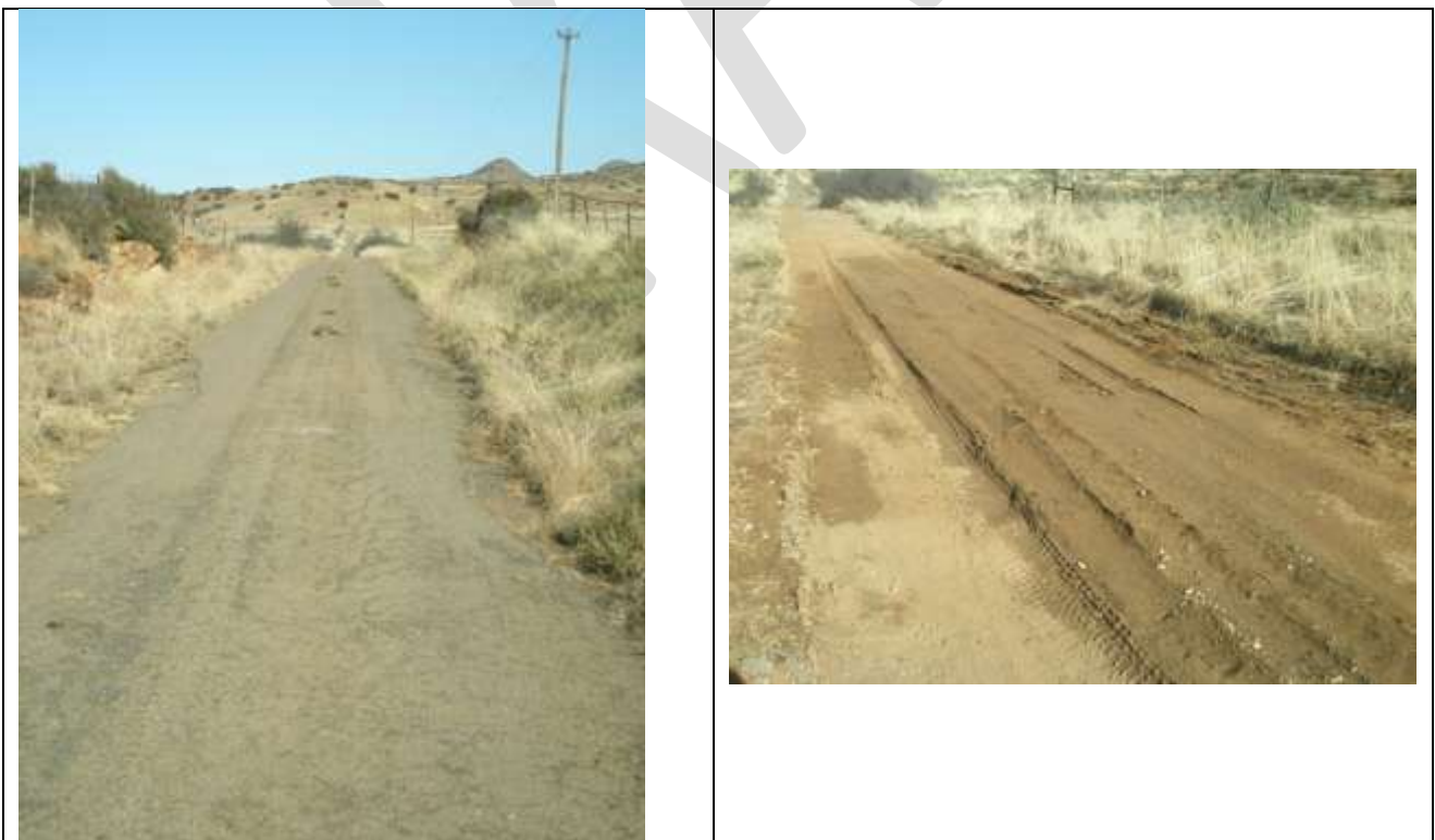
Figure 2.7. Surface condition of the access road to the quarry site
