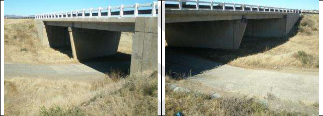
Droë River bridge: Upgrading involves a new wearing course, service/replace joint seals, and replacing balustrades with standard SANRAL detail.
