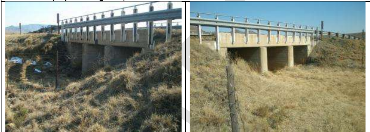
3 rd Wilwekop Spruit bridge: Widen/replace the existing bridge to suit new road alignment and cross section. Capacity improvements.
