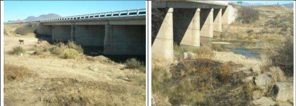
Klein Brak River bridge: Upgrading involves a new wearing course, service/replace joint seals, and replacing balustrades with standard SANRAL detail.
