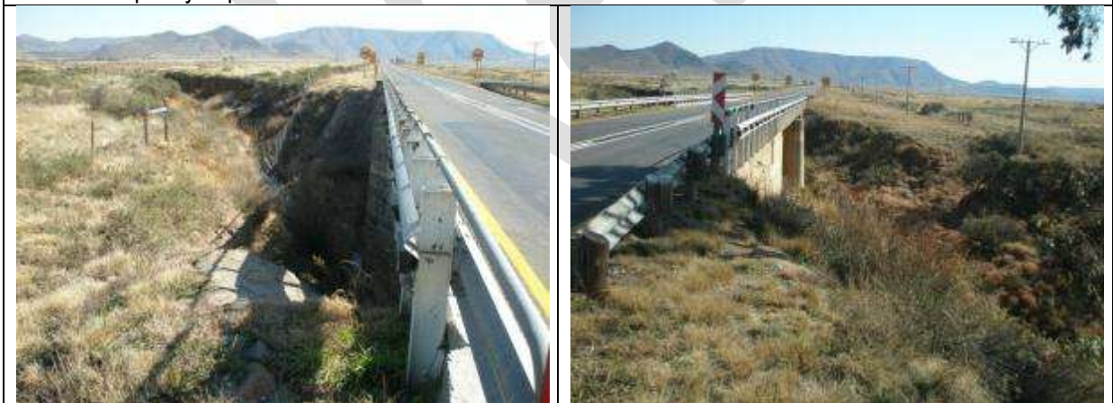
Ludlow Stream bridge: Widen/replace the existing bridge to suite new road alignment and cross section. 2 possible permanent stream deviation alternatives proposed.
