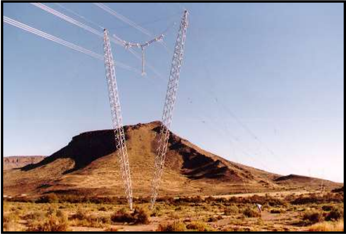
Figure 8: Guyed V structure
