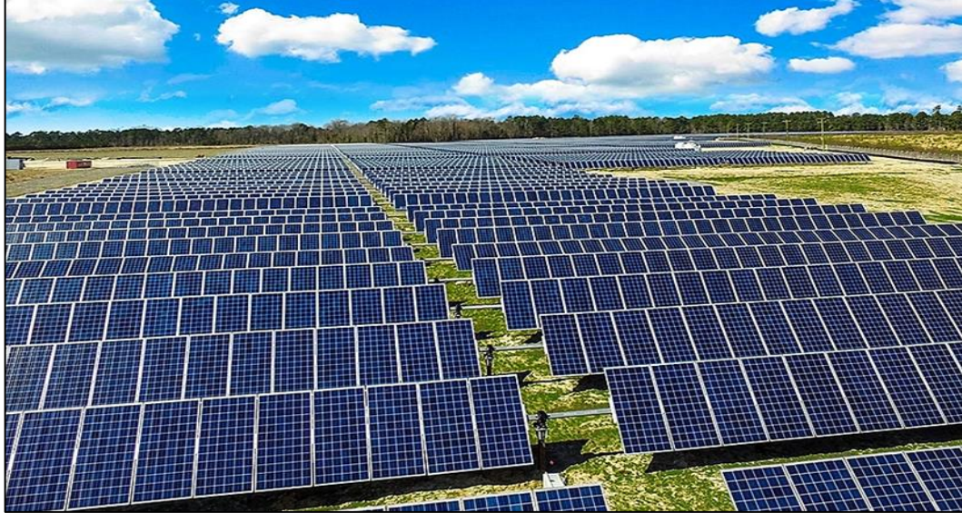
Figure 2.1: Typical example of solar PV array
