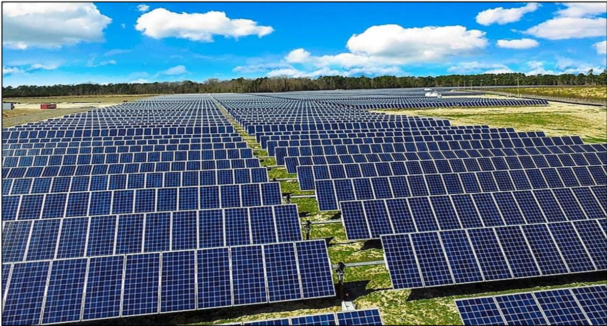
Figure 2.1: Typical example of Solar Power Plant array
