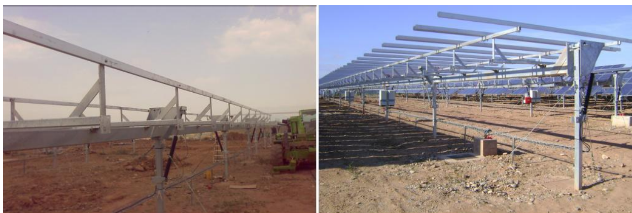
Figure 2.5: Frame, structural details (Courtesy of Igeam, 2011) The following figure shows how the structure is mounted on site.
