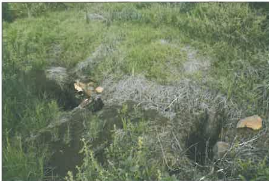
Photo 3: Evidence of an old drain near to one of the houses.
