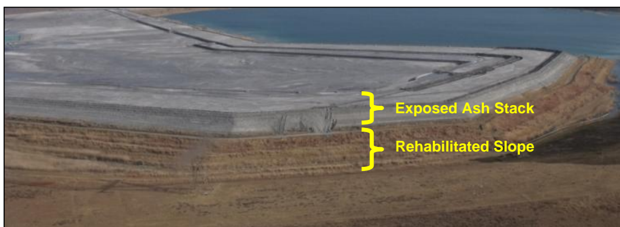
Figure 3-2: Example of an existing ash disposal site with capped and rehabilitated area in the foreground
