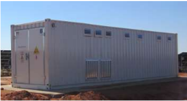
Plate 5: Typical example of inverter room (Solek, 2014)
