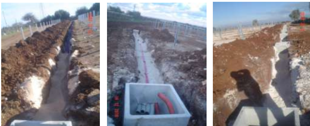
Plate 7: Typical example of internal cable trenching (Solek, 2014)
