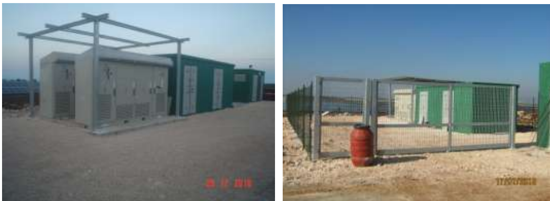
Plate 6: Typical example of on-site substation (Solek, 2014)
