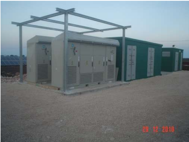
Plate 11: Typical example of on-site substation (Solek, 2014)
