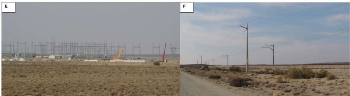
Figure 6-22:| E: Photograph of the Eskom Helios Substation; F: Photograph of the overhead electrical structures and cabling associated with the Sishen-Saldanha railway line.
