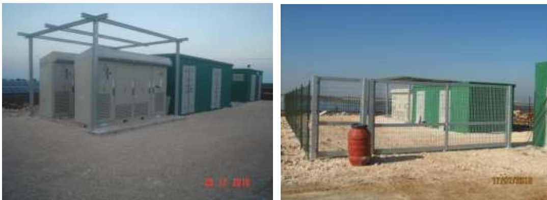
Plate 6: Typical example of on-site substation (Solek, 2014)
