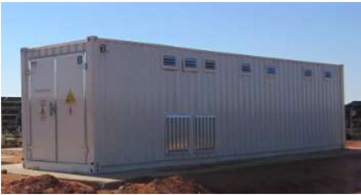
Plate 5: Typical example of inverter room (Solek, 2014)
