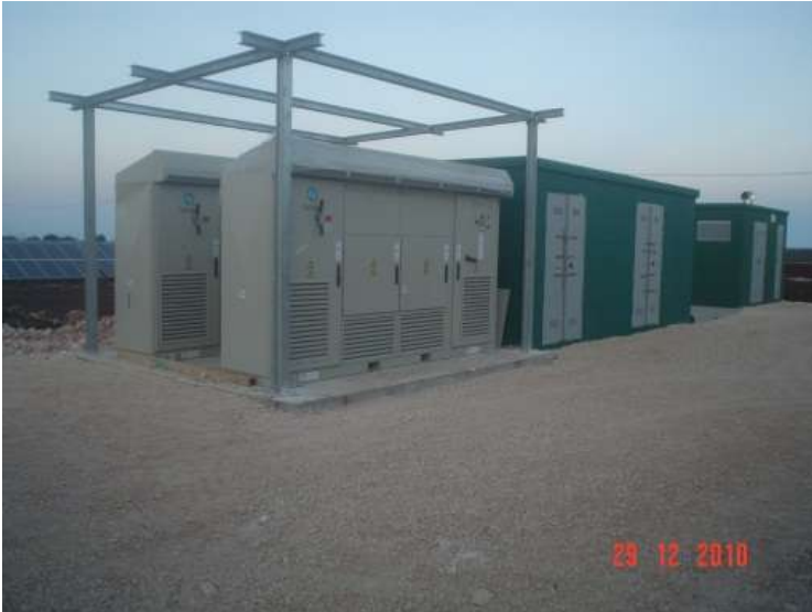
Plate 11: Typical example of on-site substation (Solek, 2014)
