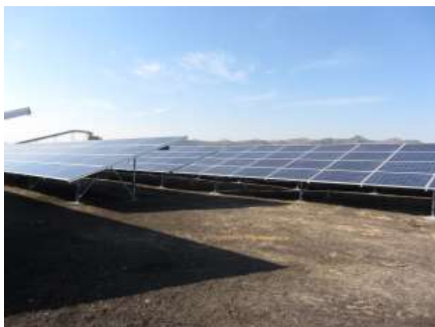
Figure 2.3: PV panels installed (RustMo1 PV Solar Facility)
