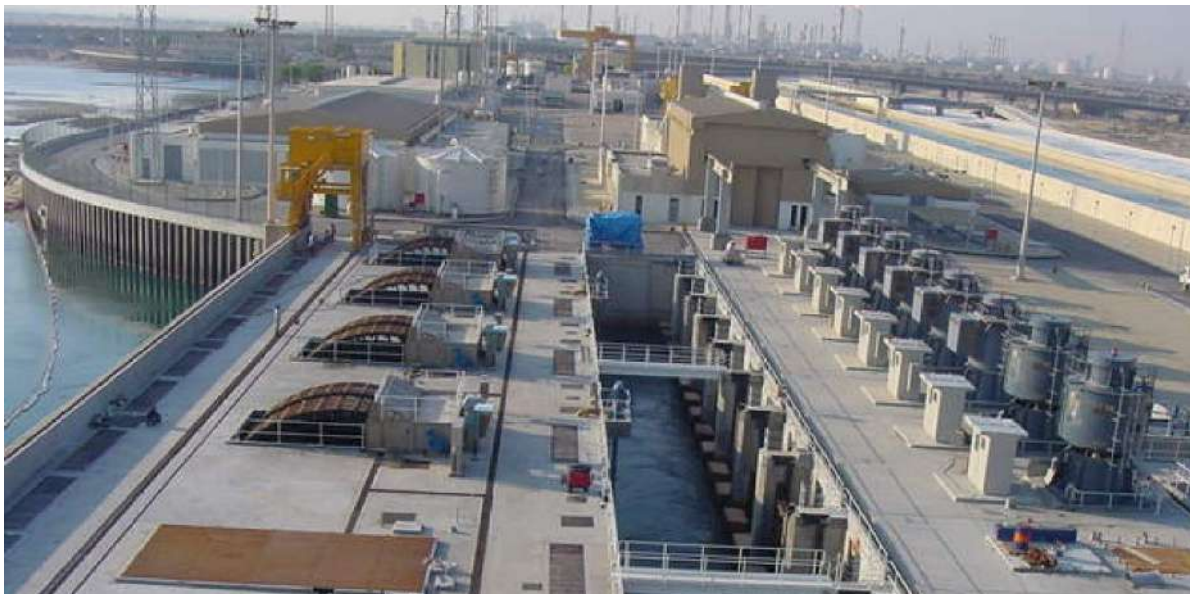
Plate 2.2: Examples of once-through cooling seawater intake infrastructure with vertical pumps on the right (Fluor, Saudi Arabia).
