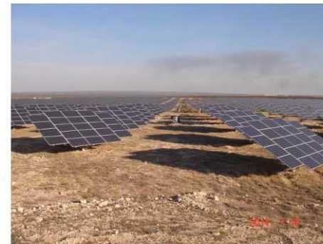
Tracking PV solar panels near Kathu, Northern Cape
