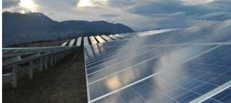
Figure 7: Fixed or rack structure PV power plant
