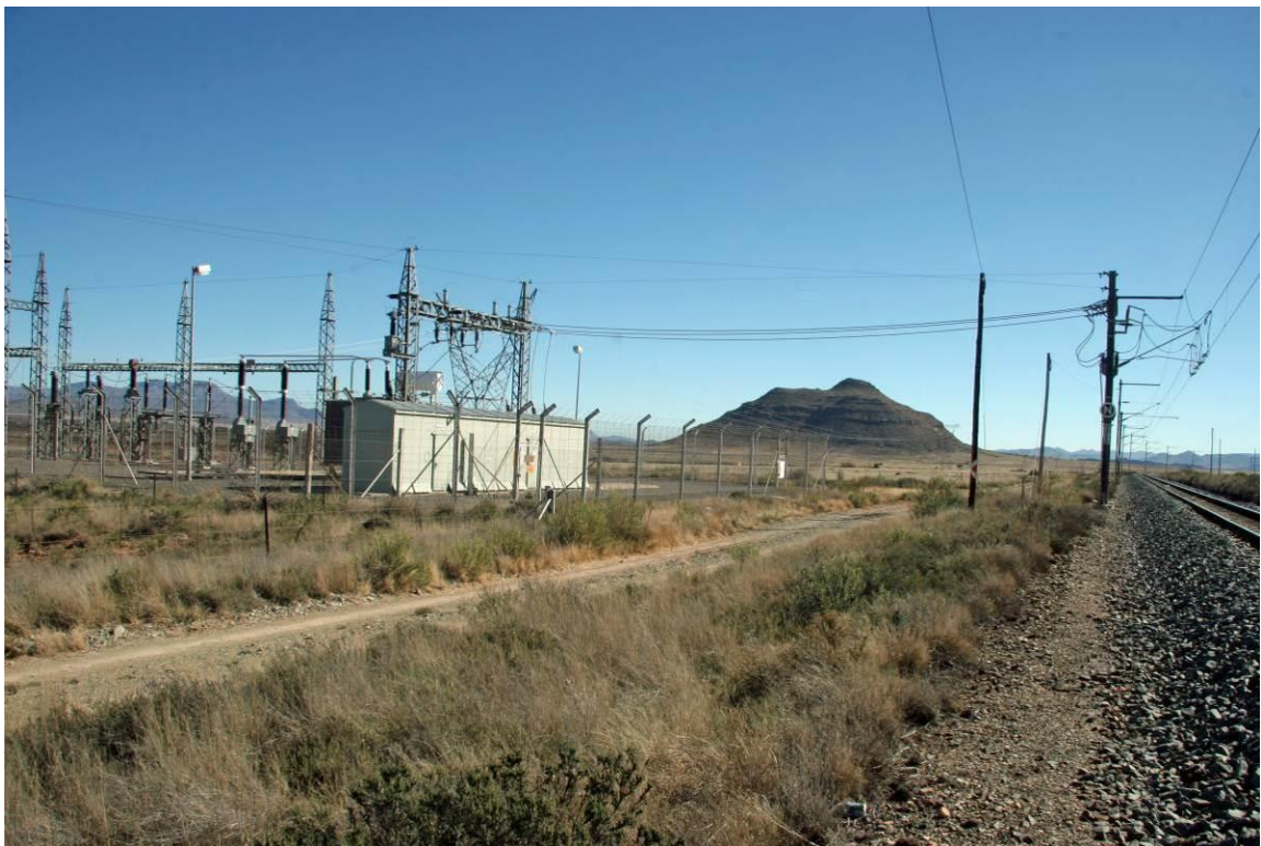
Figure 3: Views of the Collett substation adjacent to the Cradock-Noupoort railway line, where the generated electricity will be fed into the Eskom grid, indicating the Transnet service road along the railway line that could possibly be used as access road to the proposed development site.
