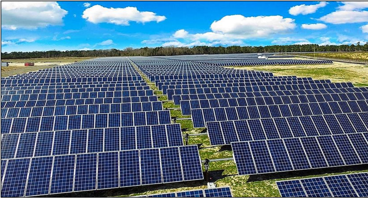
Figure 2.1: Typical example of Solar Power Plant array
