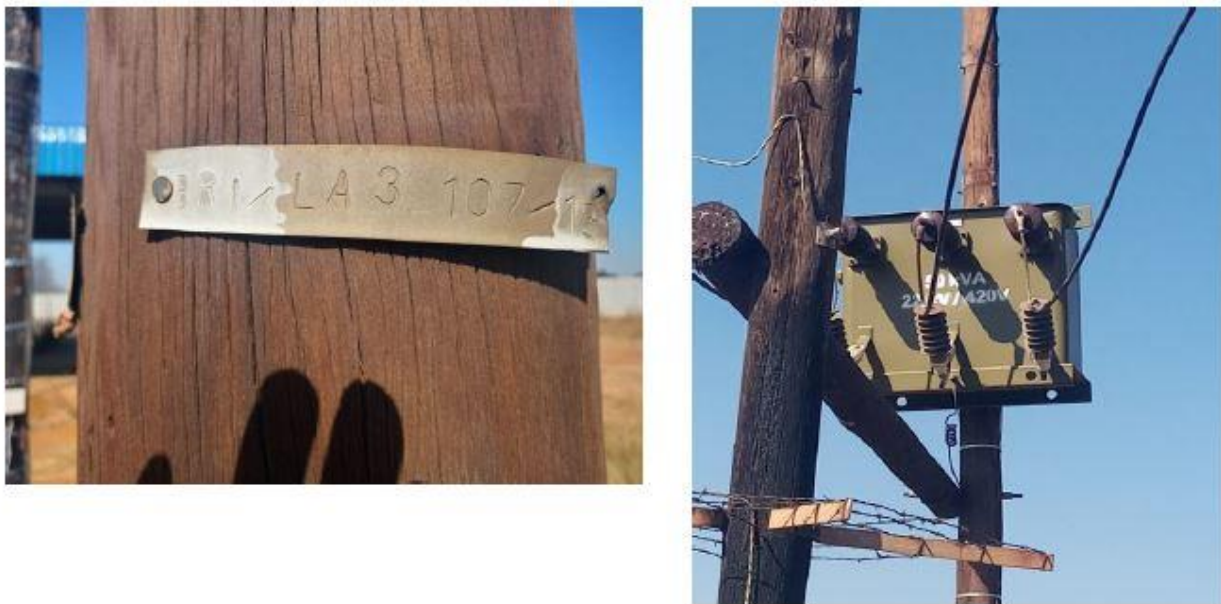
Figure 3: Eskom Pole BRI/LA3 107/13
