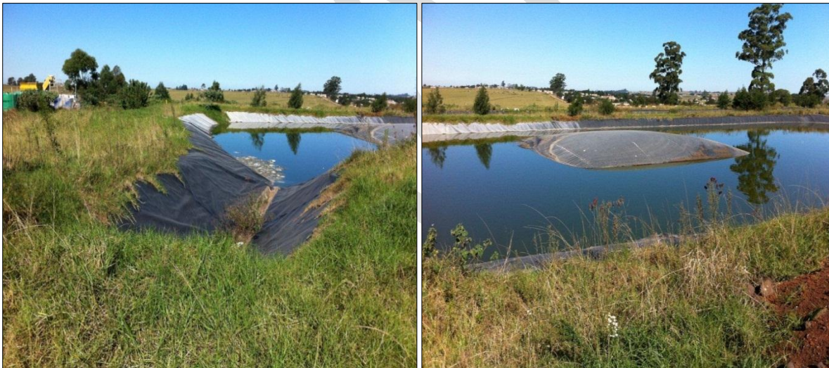
Figure 2.1 Existing oxidation ponds at St Patrick's Hospital. Left: inlet; Right: an air bubble developed indicating leakage in the lining of the pond.
