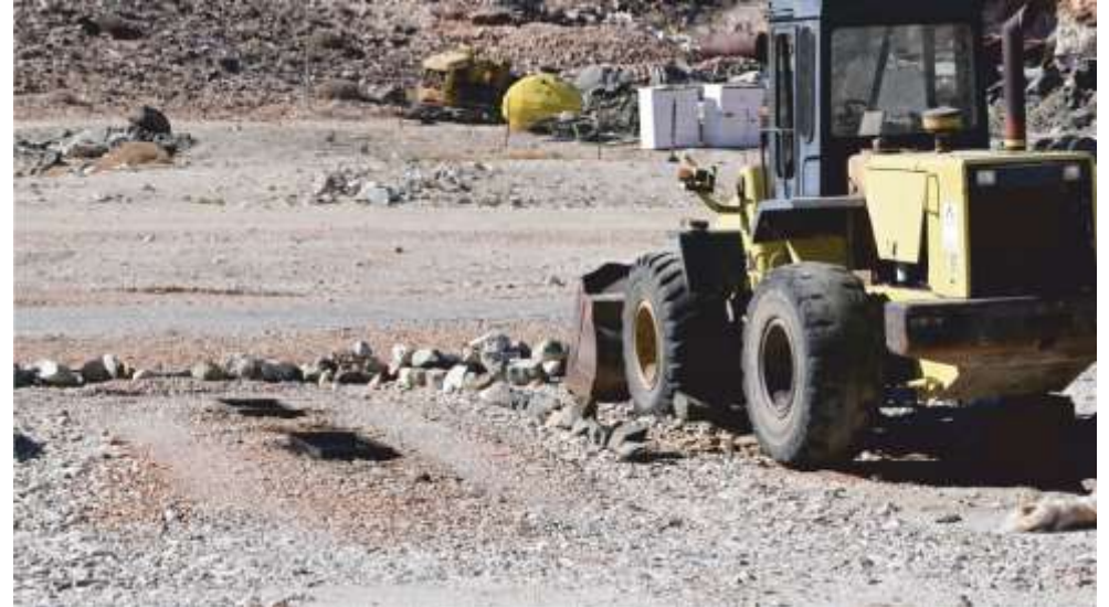
Photo 15: Drip trays in position. Needs more attention given the oil stains still on surface
