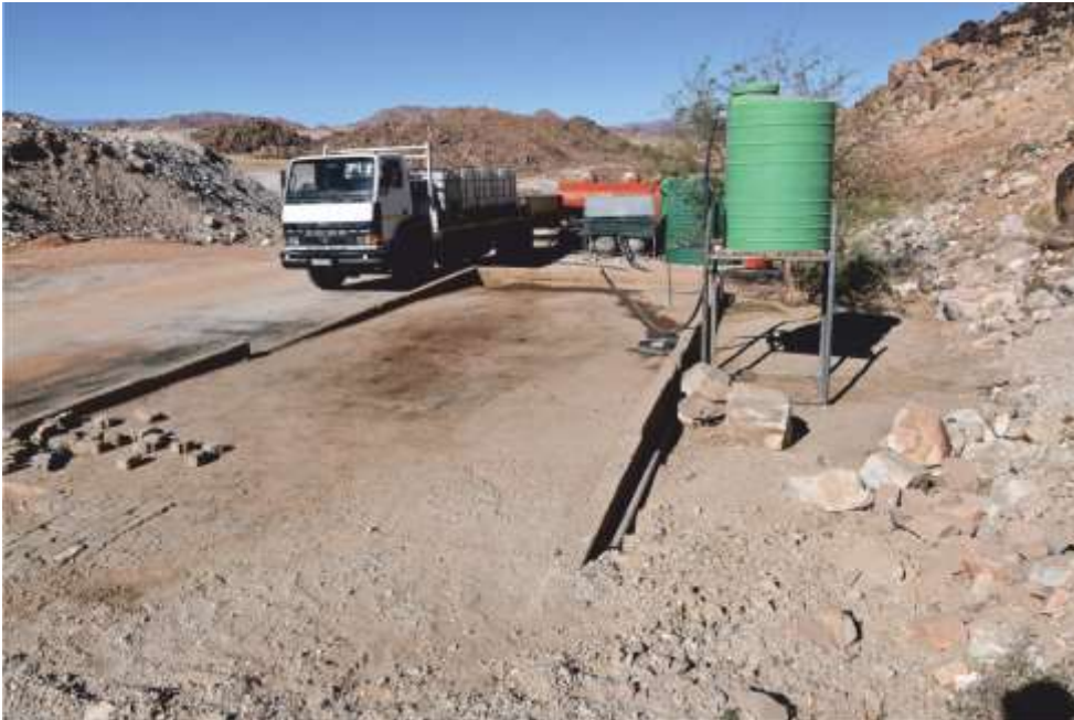
Photo 16: Wash bay facility with a very basic oil trap. Oil trap must be upgraded and covered despite very low rainfall
