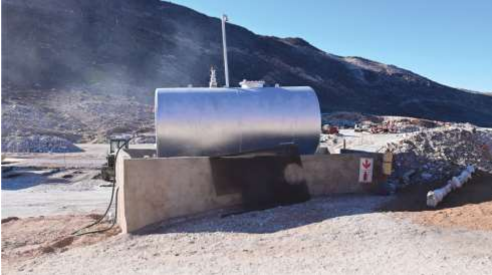
Photo 14: The bunded fuel tank. The bund was a bricked structure, but has recently been plastered at the DMRE's instruction
