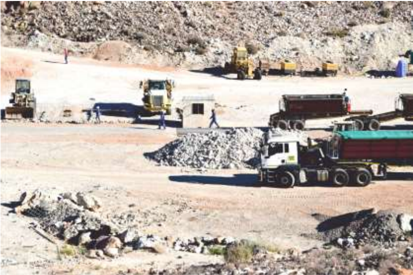
Photo 8: Weighbridge and dispatch facility
