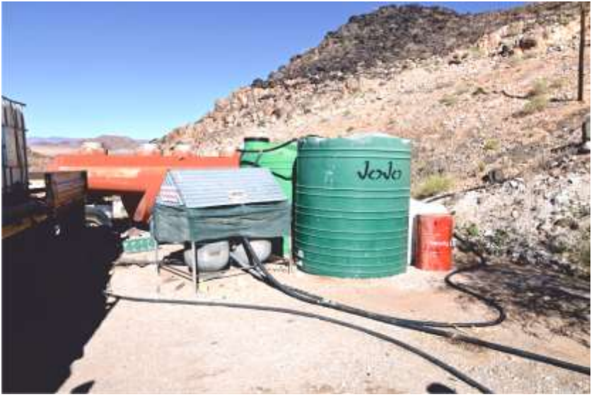
Photo 9: Small water purification plant
