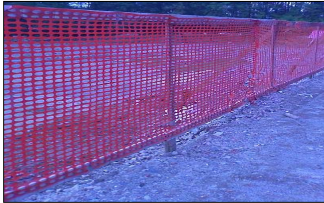
Figure 3: An example of the fence that should be placed around the boundary of the site, especially along the northern portions of the site (source: http://www.norfoss.com/construction-site-fencing/construction-site-fence.html ).
