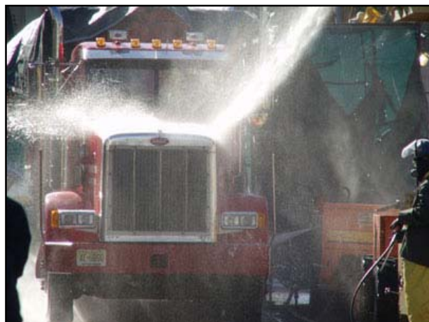
Figure 23: Illustrating an example of water runoff generated from washing vehicles that may contaminate the surrounding environment. Washing and refuelling on site must take place within the designated area in the workshop area.
