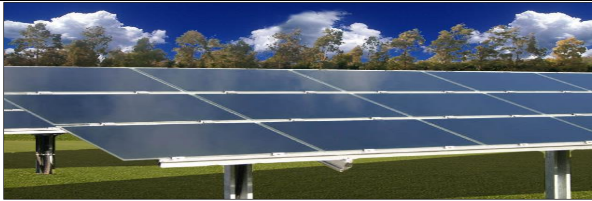
Figure 4-2: Frontal view of PV arrays mounted on fixed mounting systems.
