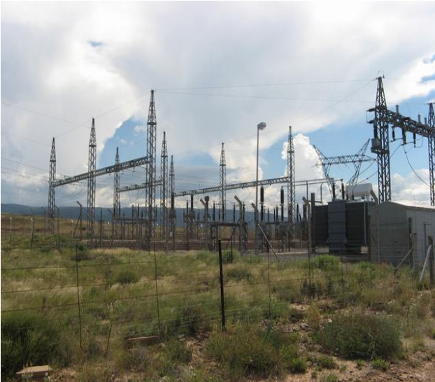
Figure 3: Drennan Traction Substation
