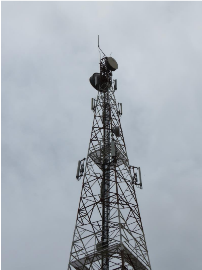
Figure 6: Typical telecom tower
