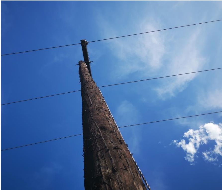
Figure 11 Electrical infrastructure onsite
