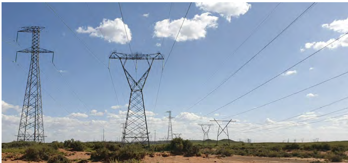
Figure 5: Multiple overhead power lines converge on the Eskom Hydra Main Transmission Substation, mostly without bird flight diverters
