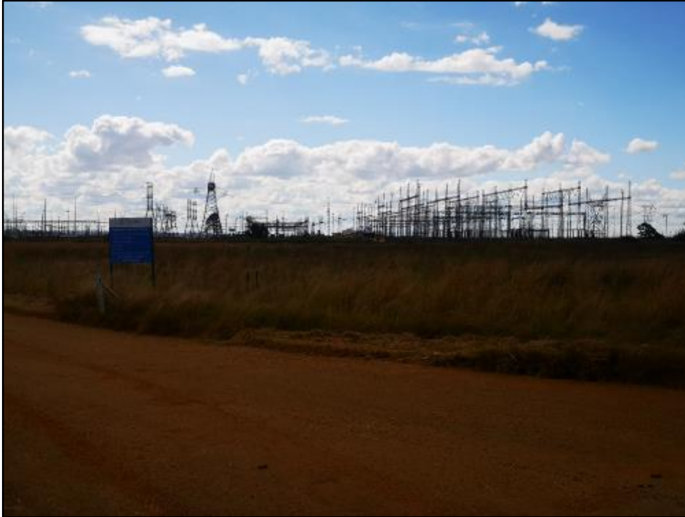
Photograph 3.5: Eskom Mercury Substation
