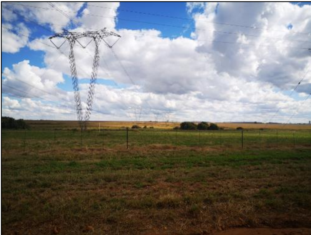
Photograph 3.9: View looking west from Vermaasdrift Road towards Kleinfontein and Biesiefontein PV SEF sites
