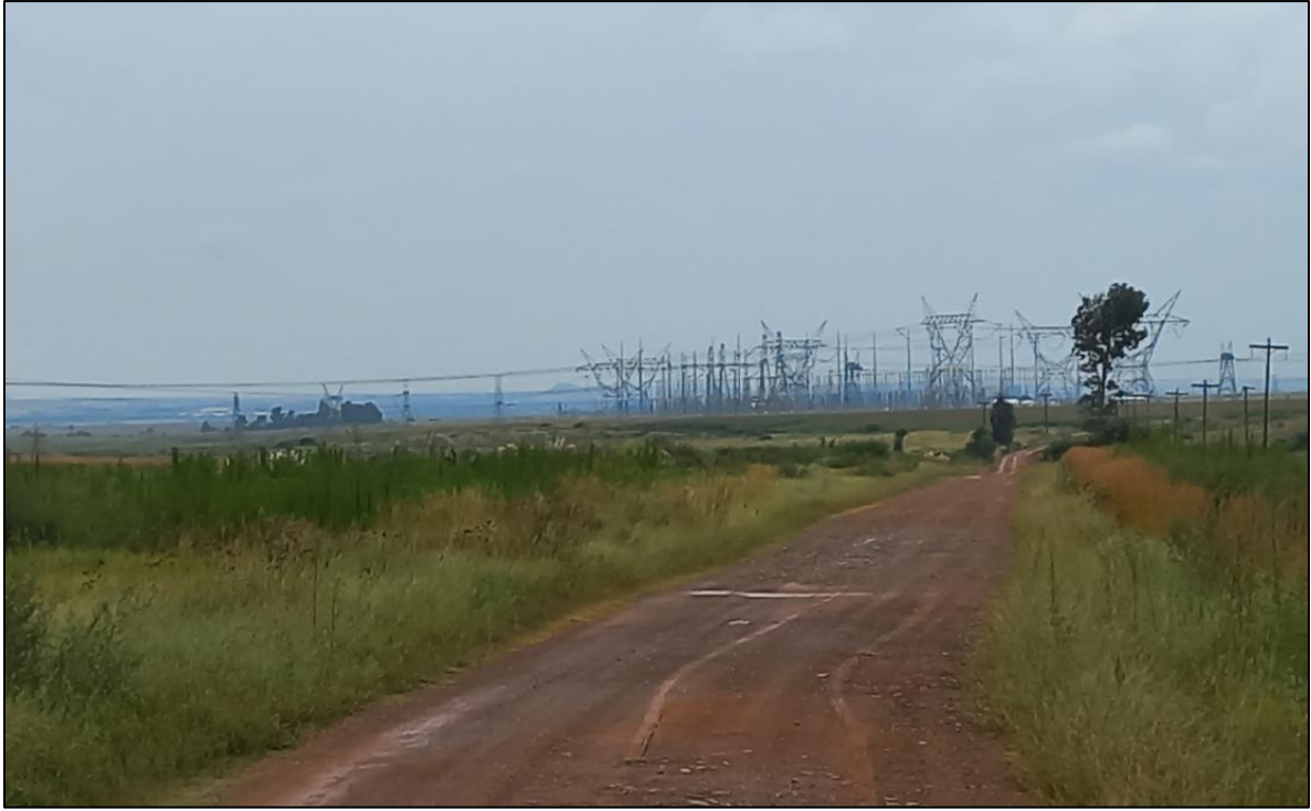
Figure 11: Photograph of the Eskom Mercury Substation.
