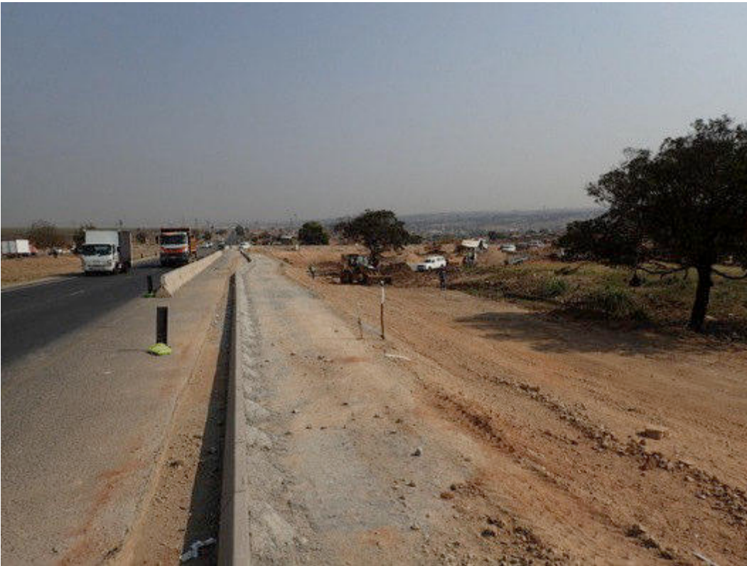
Figure 28 View of Site 2 towards the northwest with additional road infrastructure and storm water structures under construction
