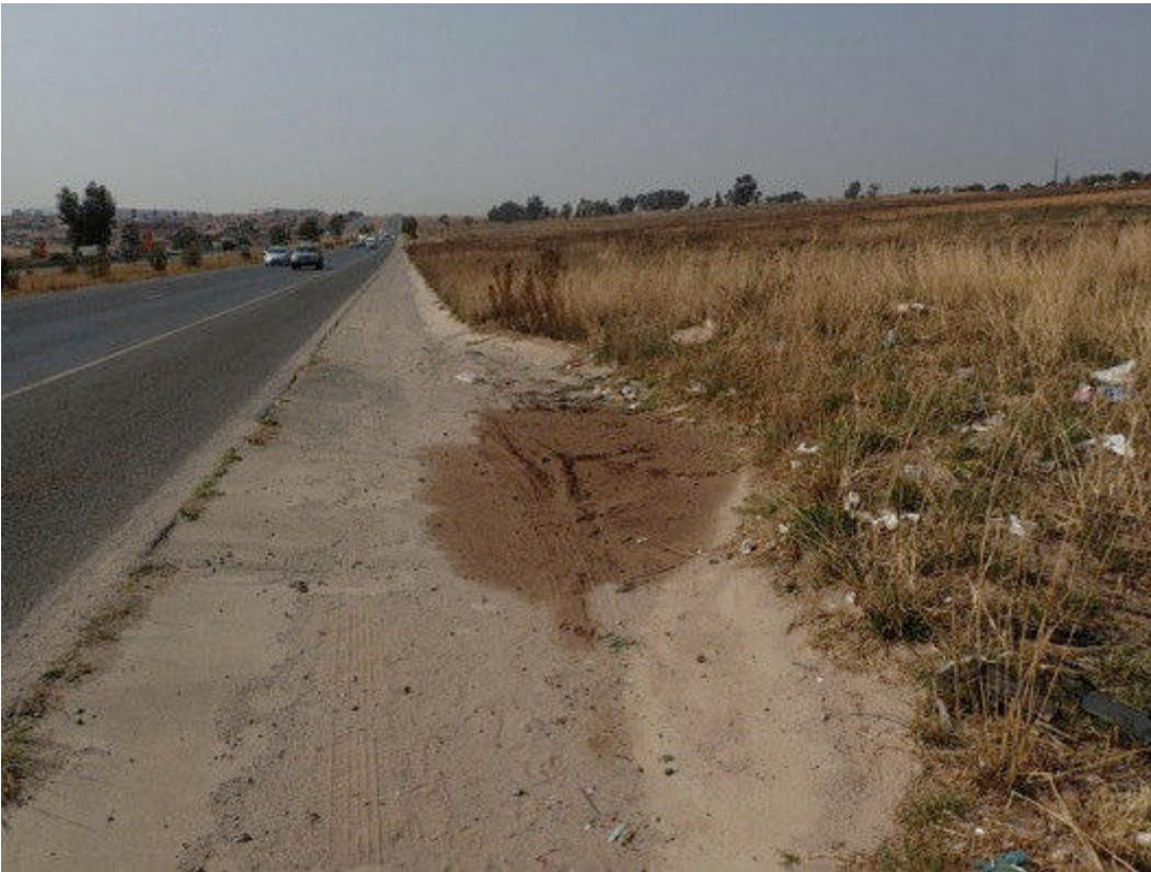
Figure 41 Blocked storm water inlet on Allandale Road on Site 2
