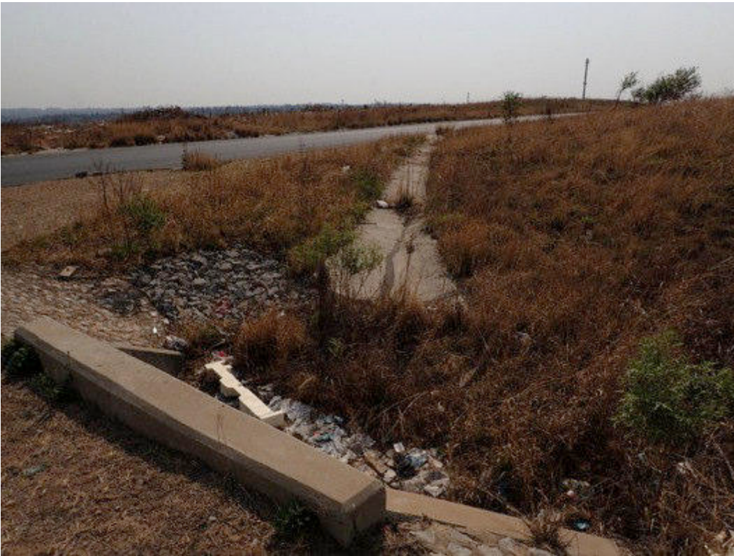
Figure 46 Storm water inlet under the access road to the Waterfall Cemetery
