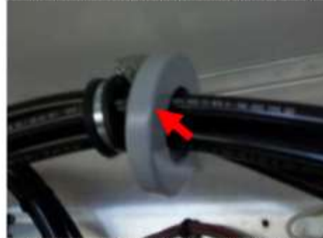
DC side High Power Wiring for EMI shielding
