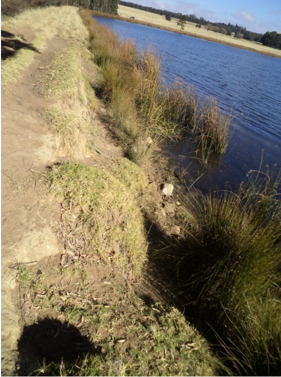
Photograph 3 Crest Upstream Erosion
