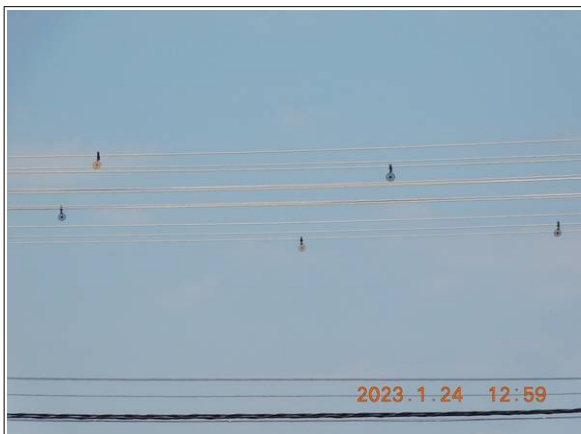
Photograph 9: Bird diversions on powerlines, indicating previous fauna mitigation measures implemented on
