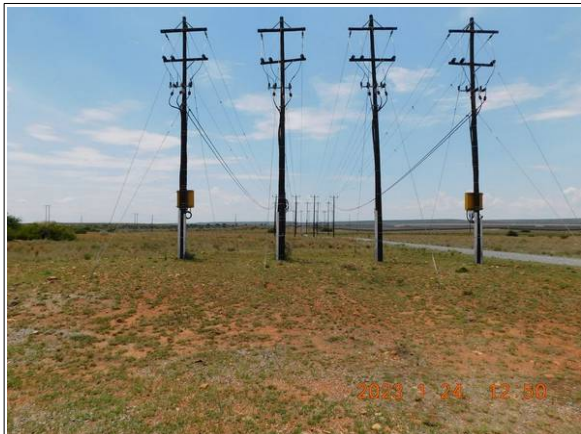
Photograph 7: Overhead powerlines from Lesedi North to the substation; originally planned as underground cables
