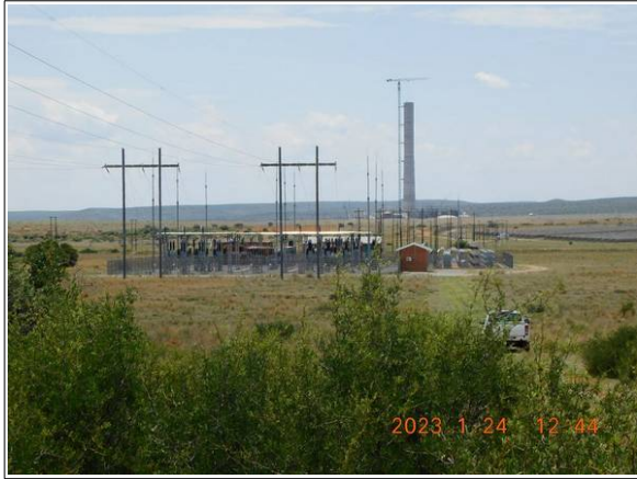
Photograph 5: Fenced-off substation with surrounding grasslands; lines feeding into the Eskom grid in the foreground
