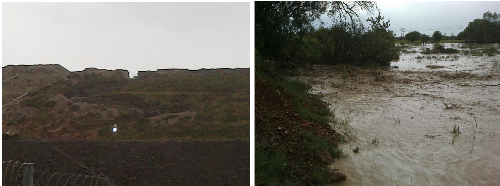
Failure of Tailings Storage Facility's walls with resultant spillages of toxic and radioactive slurry on farmland and into the Koekemoerspruit
