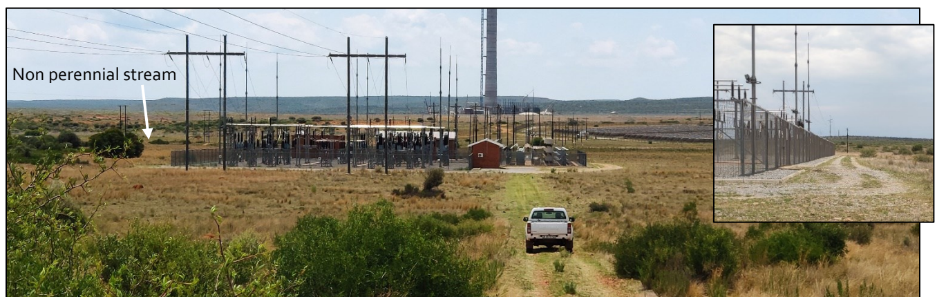
Photo plate 4: View of the substation, looking northwards, in a grass dominated landscape
