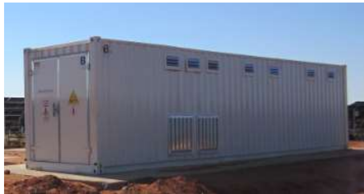
Figure 7: Typical inverter room
