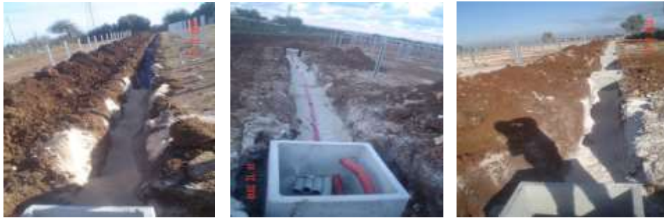
Figure 9: Typical cable trenches.
