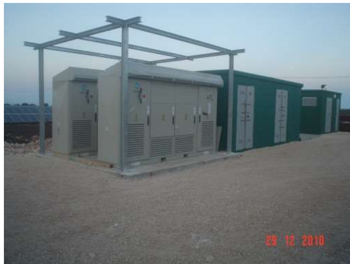
Figure 20 : Typical on-site substation
