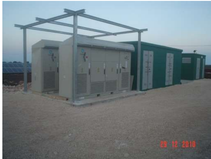
Figure 20 : Typical on-site substation
