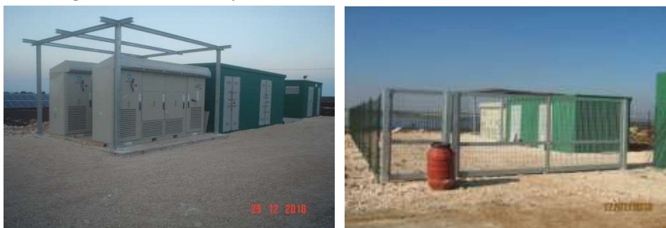
Figure 8: Typical on-site substation footprint
