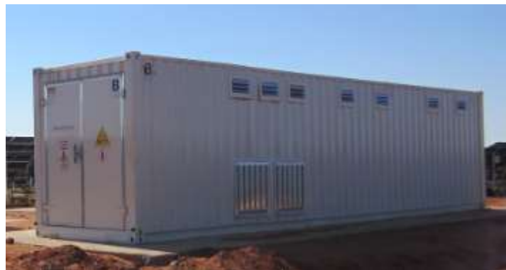
Figure 7: Typical inverter room
